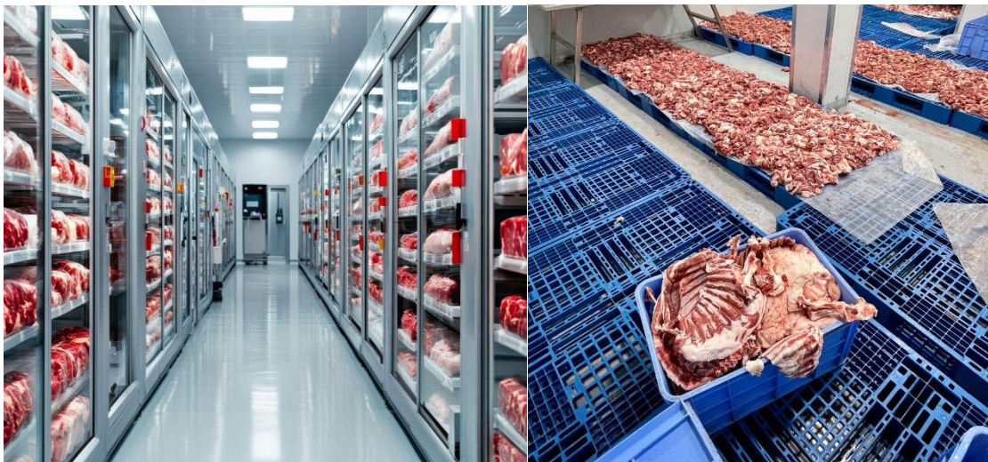
Figure 1. Cold Storage and Refrigeration Systems for Meat Preservation Cold Storage and Refrigeration
