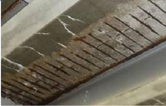
Figure 1. Defects and damage caused by moisture retention
