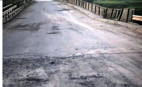
Figure 2. Defects and damages caused by loads and structural wear and tear
